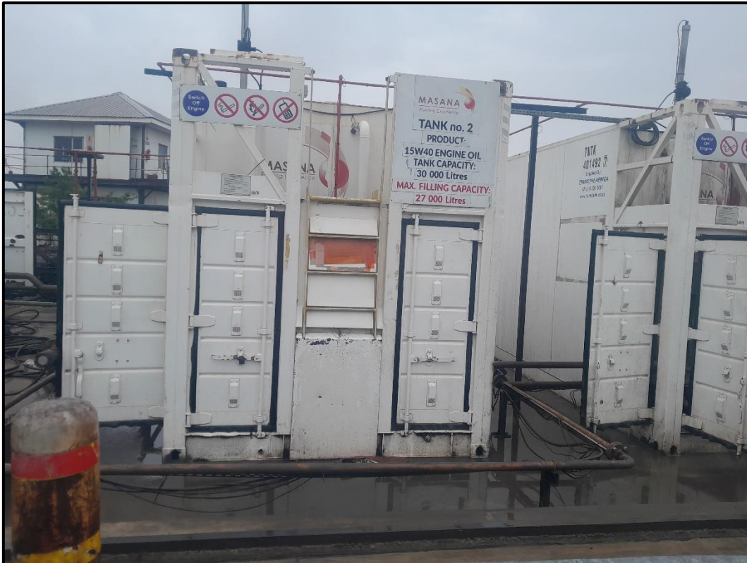
Figure 5. Confirmation of bund capacity of fuel storage facility required.
